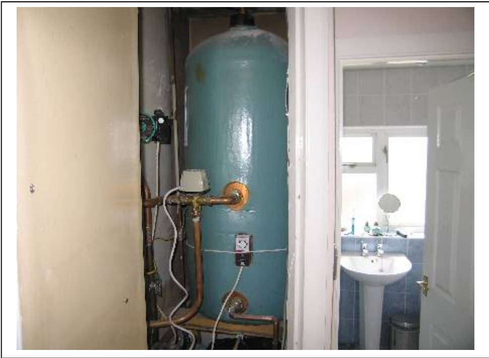
Hot water cylinder.
